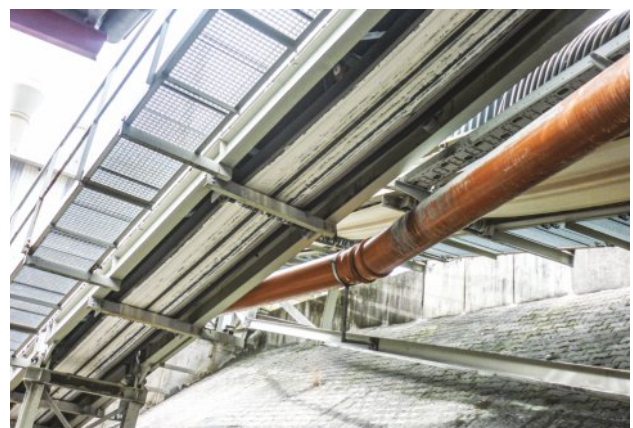
Before: Caking on the rollers leads to misalignment and damage to the belt
