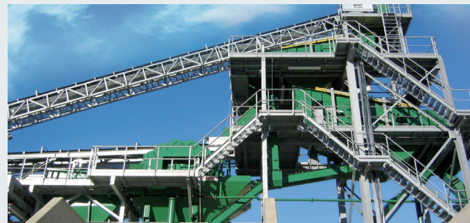
STICHWEH preparation plant with DOUBLE-DECK SCREENING MACHINE VS 18/50 DOUBLE-DECK SCREENING MACHINE VS 21/60 Bucket wheel E 4009 LA Dewatering screen Eb 12/35-03
